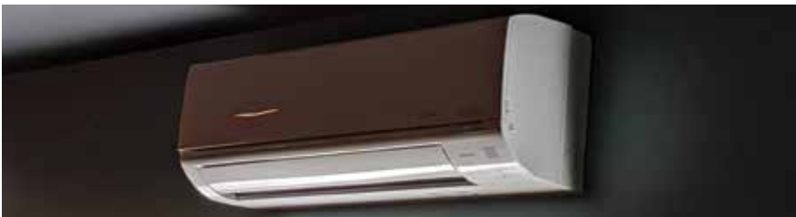
Upstairs Worship Area Air Conditioning Fall 2019
